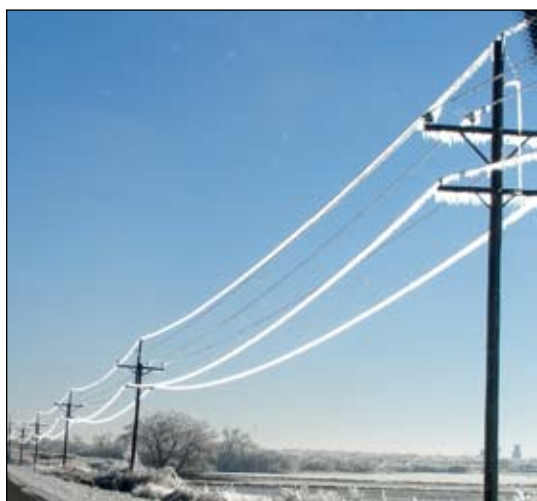
Power lines coated in ice continued to cause outages up to a week after the storm.
