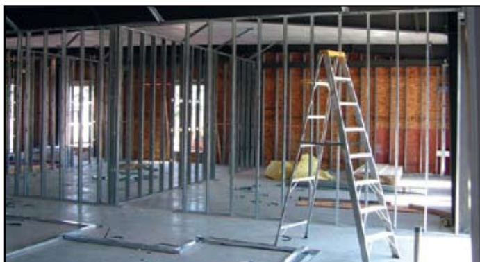
Construction of the Western Cooperative addition is scheduled for completion in fall 2008.
