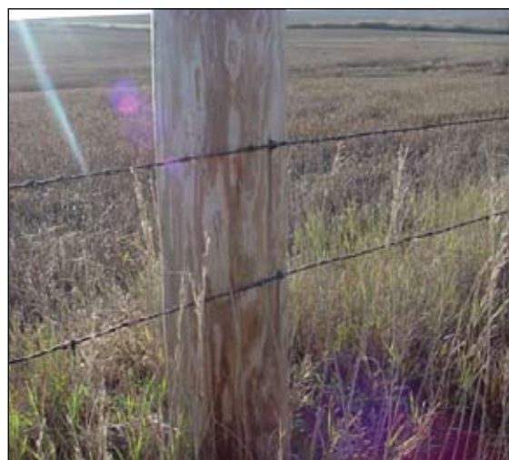
Barbed wire attached to a power pole on Western's system can be hazardous to our linemen.
