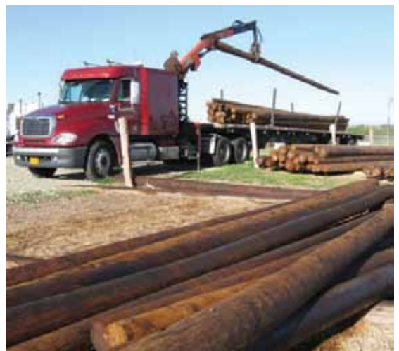
The FEMA project will reconstruct 430 miles of line, which includes approximately 8,600 poles.
