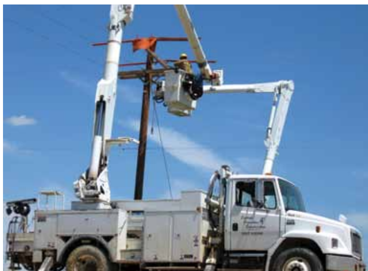
Line crews from Texoma Powerline, Inc., and Custom Powerline Construction were hired to aid in the rebuilding process.
