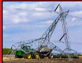
NO-TILL AIR DRILL DAMAGED HIGH VOLTAGE TRANSMISSION EST. REPAIRS $99,995*
